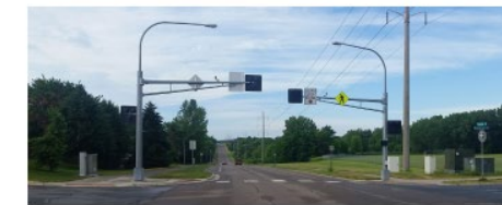
High-Intensity Activated Crosswalk Beacon
